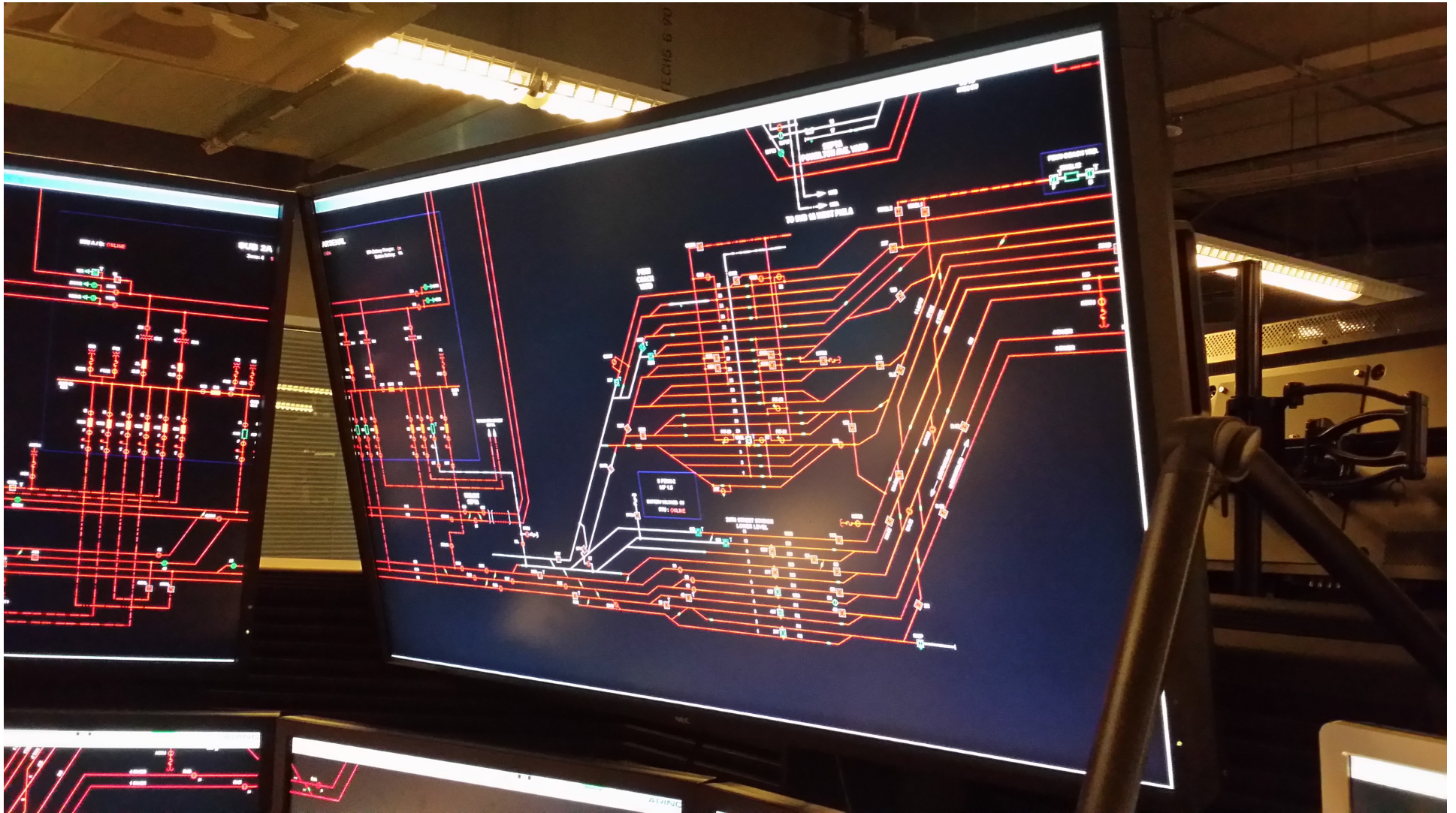
Inside the Amtrak Control Facility. These are Overhead Power Monitoring Displays (Live wire is shown as Orange). (Photo: Geert Marien)
