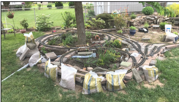
Track roadbed using cement products and stone slabs with the wiring conduit exposed and the finalized track plan
